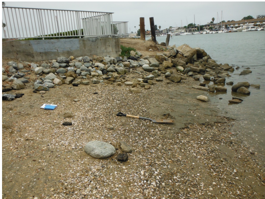
Photograph C-2. Looking south from the sandy beach towards the existing bulkhead and riprap embankment. The shovel demarcates the location of the excavated soil pit.
